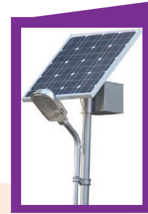
Solar powered lighting
